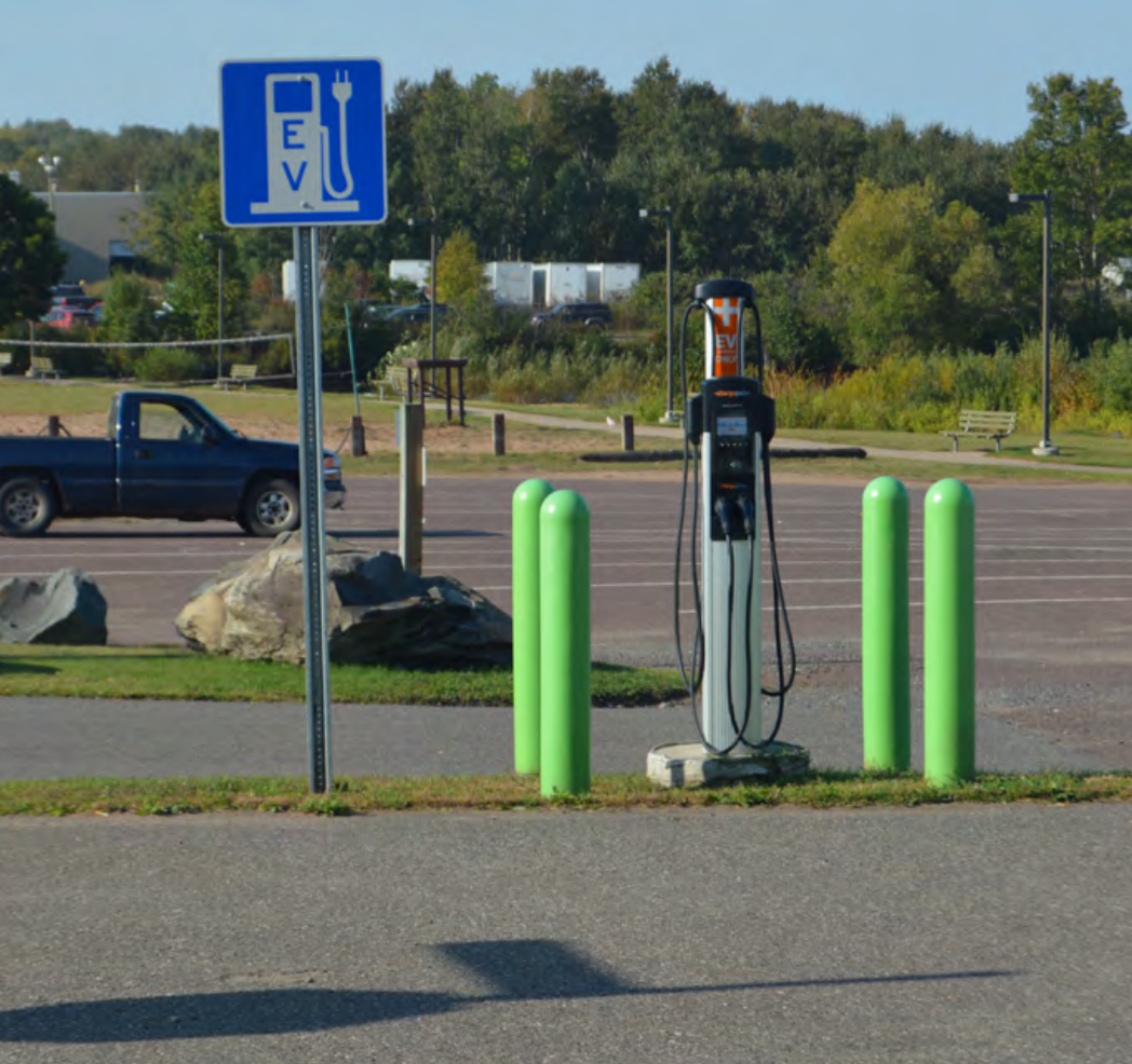
FIGURE 5.2 - EV CHARGING STATION
